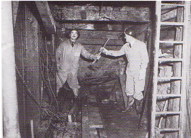
Photo 2 Alan and SEC engineer during the tunneling of power station cooling water conduits in a soft ground adjoining Yallourn Open Cut
